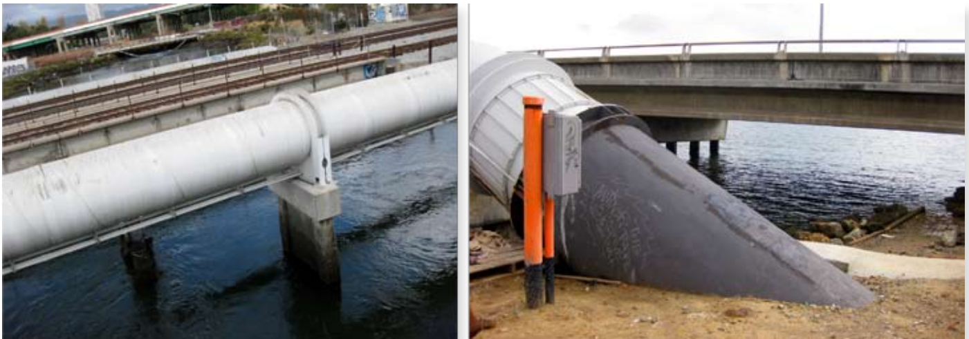
7th Street Flood Control Station pumpworks
